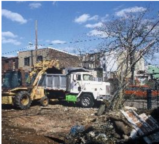
Major trash, debris, and weed removal
